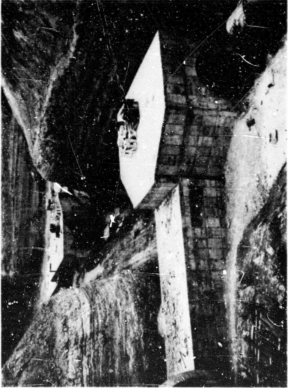
Fig. 13. Backfill around concrete blastlock structure and below haunch of steel-plate tunnel, Titan I facility
