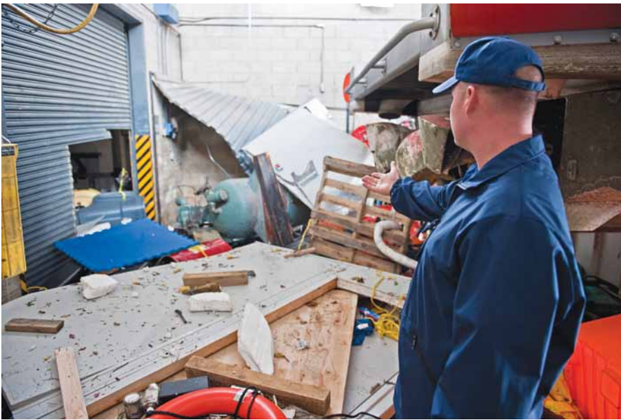
Chief Petty Officer Jeremiah Grey, Station Sandy Hook's engineering petty officer, shows the destruction in the boathouse caused by flood waters after Hurricane Sandy. U.S. Coast Guard photo by Petty Officer Luke Clayton.
