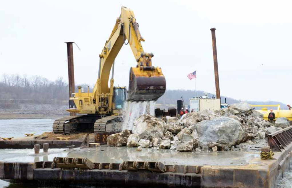
Crews work to remove the rocky obstructions during the low water operations near Thebes, Ill., in 2012. Photo courtesy of the U.S. Army Corps of Engineers, St. Louis District-MVS, photo by Romanda Walker.
